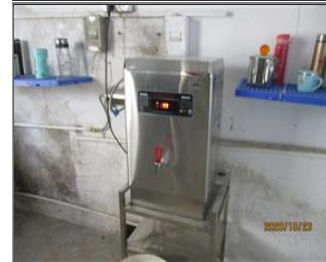
Photo of the sanitary facilities Potable water.JPG
