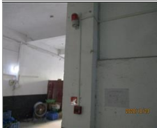
Photo of fire safety equipment Fire alarm.JPG
