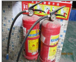
Photo of fire safety equipment Fire extinguishers.JPG
