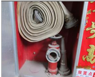
Photo of fire safety equipment Fire hydrant.JPG
