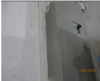
Photo of non-conformity NC 7.13 No warning sign posted for the electric boxes.JPG
