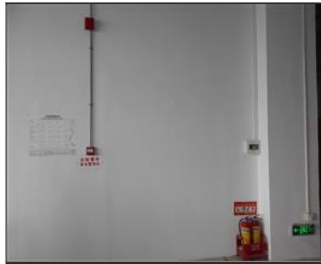
Photo of fire safety equipment Fire equipment.JPG
