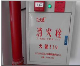
Photo of fire safety equipment Fire hydrant.JPG
