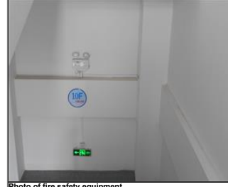
Photo of fire safety equipment Evacuation sign and emergency light in staircase of production building.JPG
