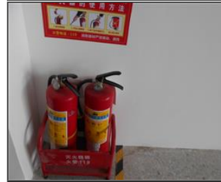
Photo of fire safety equipment Fire extinguishers.JPG
