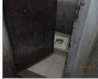
Photo of the sanitary facilities Toilet area for worker.JPG
