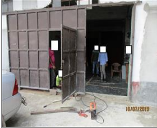
Photo of non-conformity Final exit door made outward.JPG
