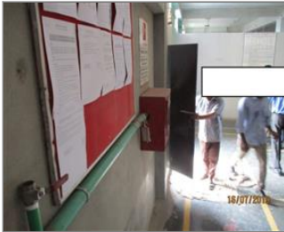
Photo of non-conformity Inward opening door found at final exit from the building.JPG
