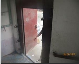
Photo of non-conformity 7.1 Second exit door made outward.JPG
