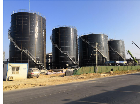
Sinopec High Salt Wastewater Treatment Project
