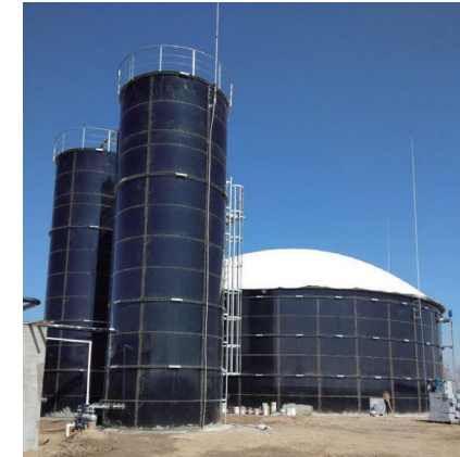
CSTR Reactor + IC Reactor in Shanghe, Jinan
