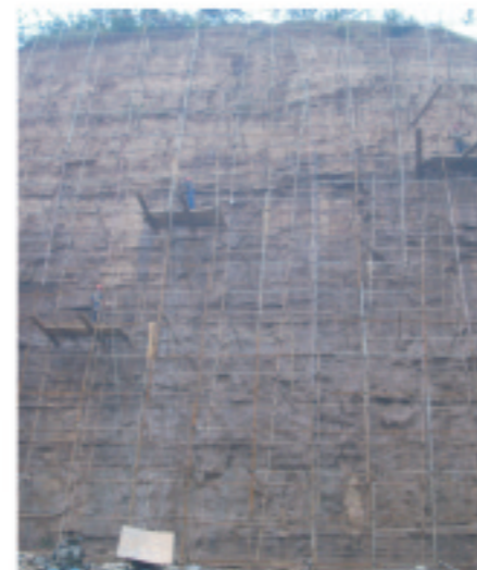
Yulong FRP Anchor Bolt used to reinforce the slope in the Fire Brigade Headquarters of Yiling District Yichang
