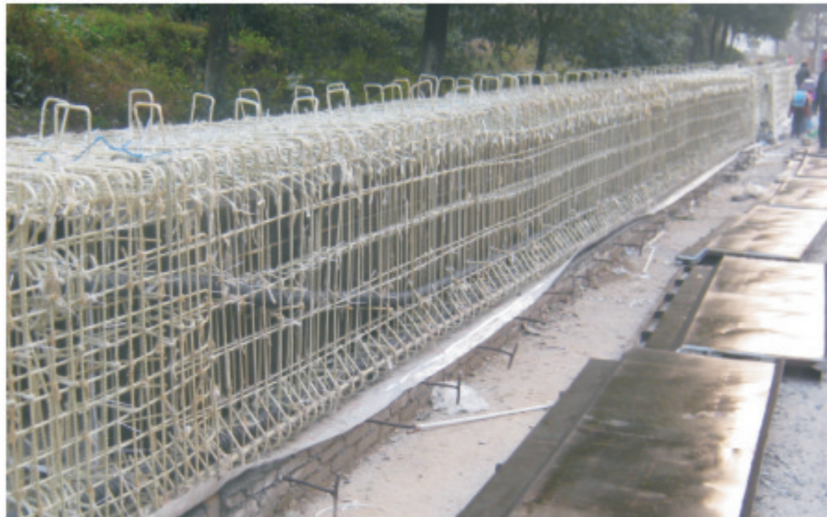
Yulong FRP rib materials used in Songshuao Bridge in Zigui Yichang (20-meter Prestress Hollow Slab)
