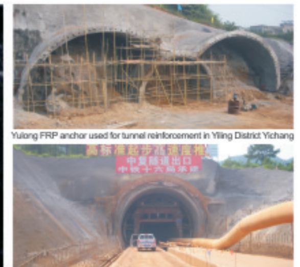
Yulong FRP anchor used in tunnel construction in Longyan in Fujian Province
