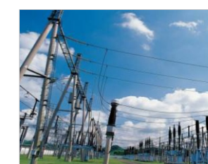
■ 配电变压 Power Distribution
