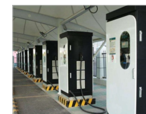
■ 充电站 (桩) Charging Station (Pile)
